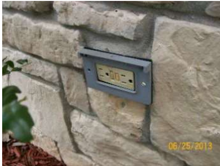
Receptacles missing covers on the front and rear of structure.
