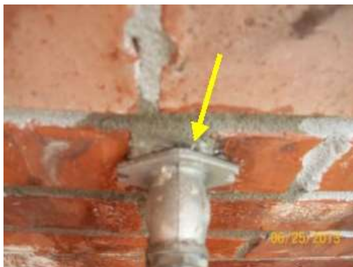
Faucet on front east of door Appears to be damaged/leaking in the wall. Recommend review and repair by a qualified plumber.
