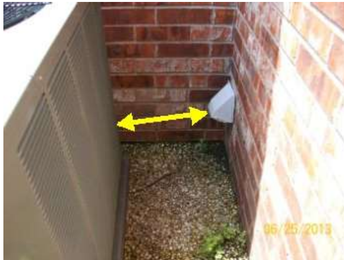
Dryer vent within 3 feet of exterior condensor.
