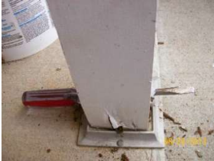
Support post on the rear of the structure in rotten on the bottom.
